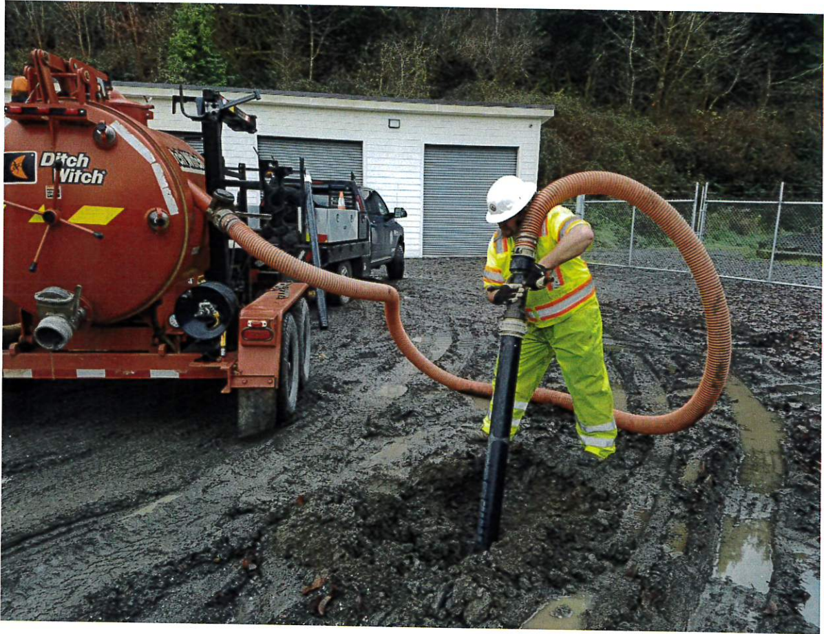
Boom not deployed, notice all the weight of the suction line is on the operator's shoulders.
